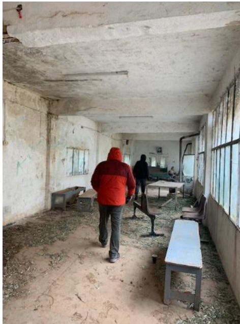
Figure 3: Sample of Jerash Nursery buildings require refurbishment
